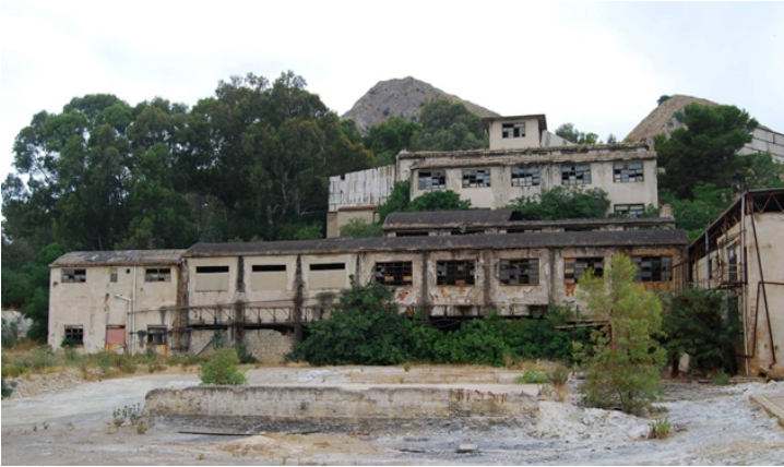
Flotation Plant yet to be restored
